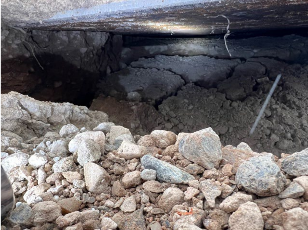
PHOTO 2 – SUBGRADE EROSION UNDERNEATH STEEL PLATE
