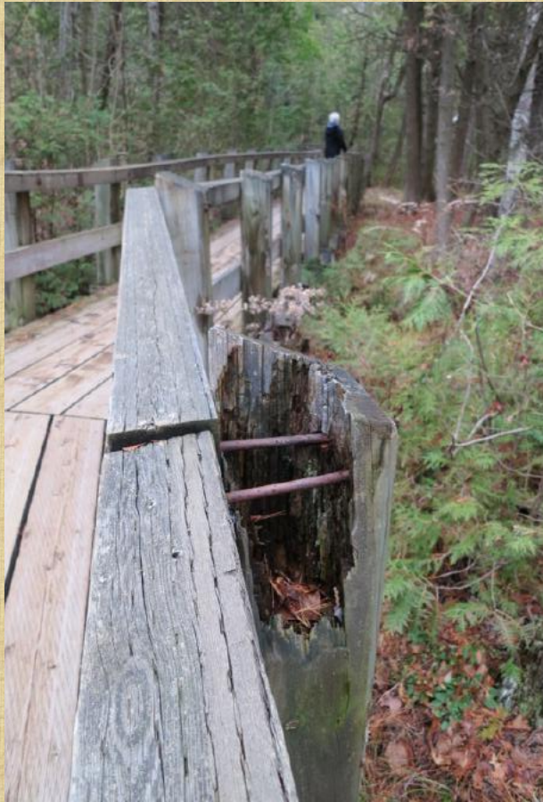
Lack on routine inspection and maintenance.
