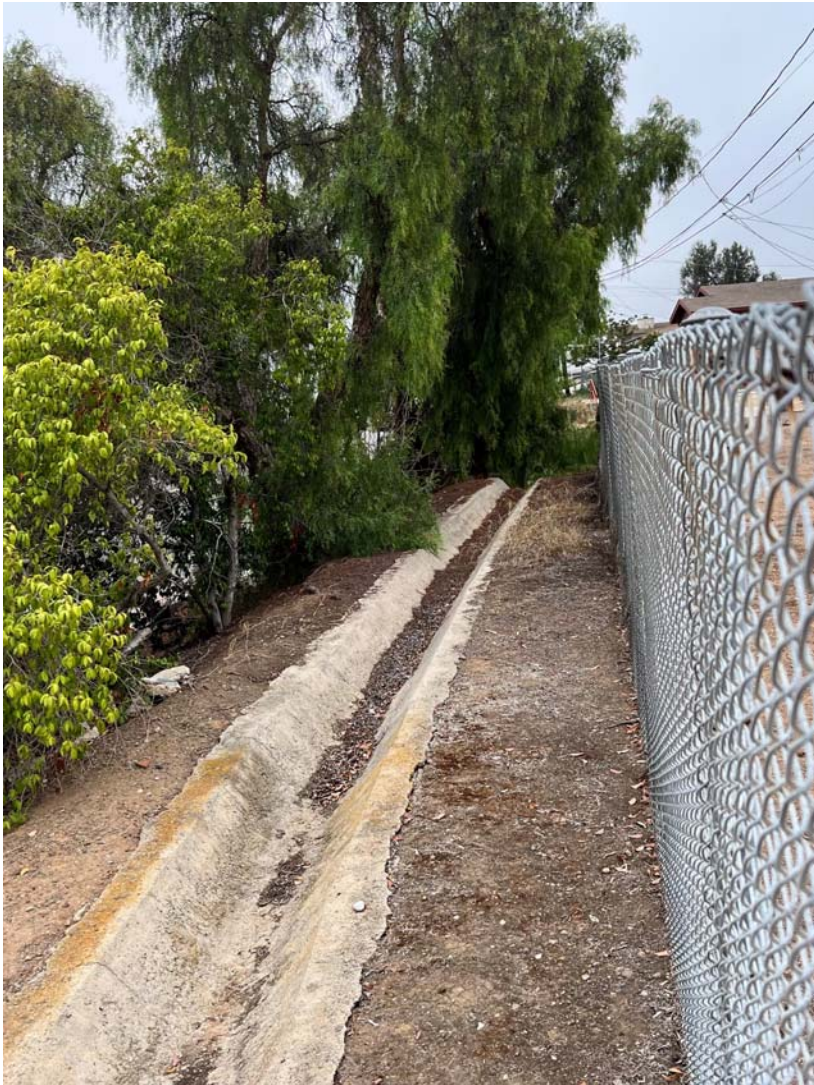
Brow ditch east of Orange Street cul-de-sac
