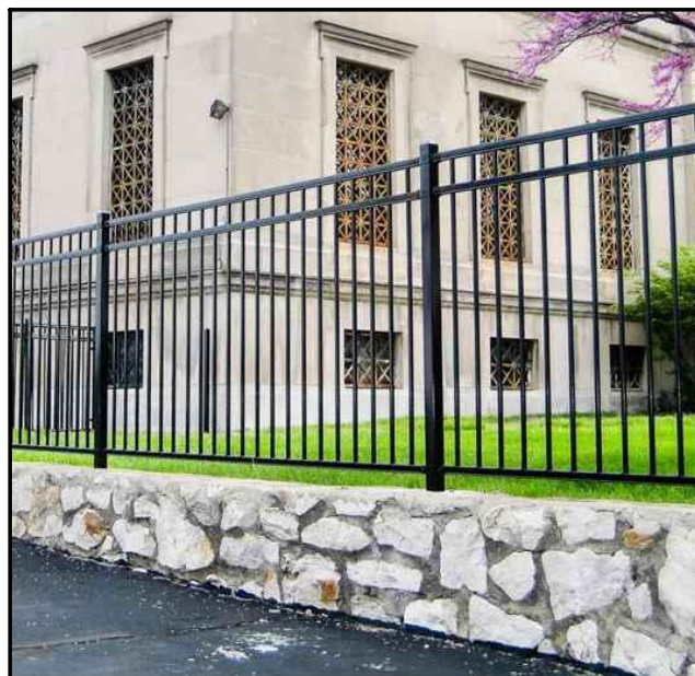
POOL FENCE: AMERISTAR MONTAGE PPP; 48" HT.
