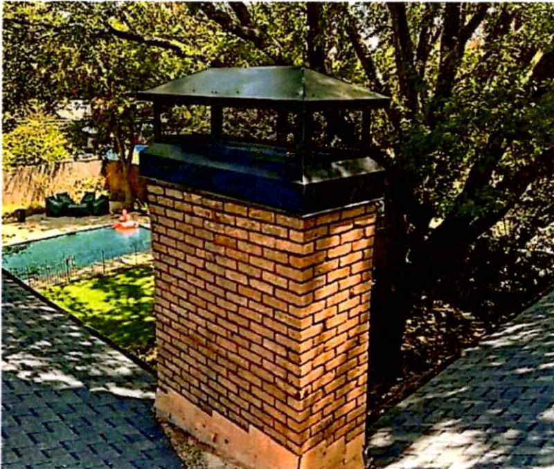
Kitchen Chimney After
