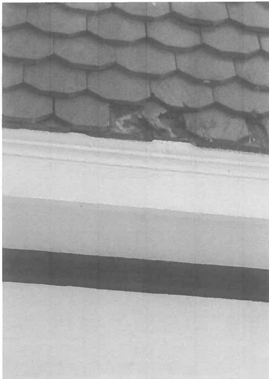
(5) DAMAGED FISH SCALE CEDAR SHINGLES
